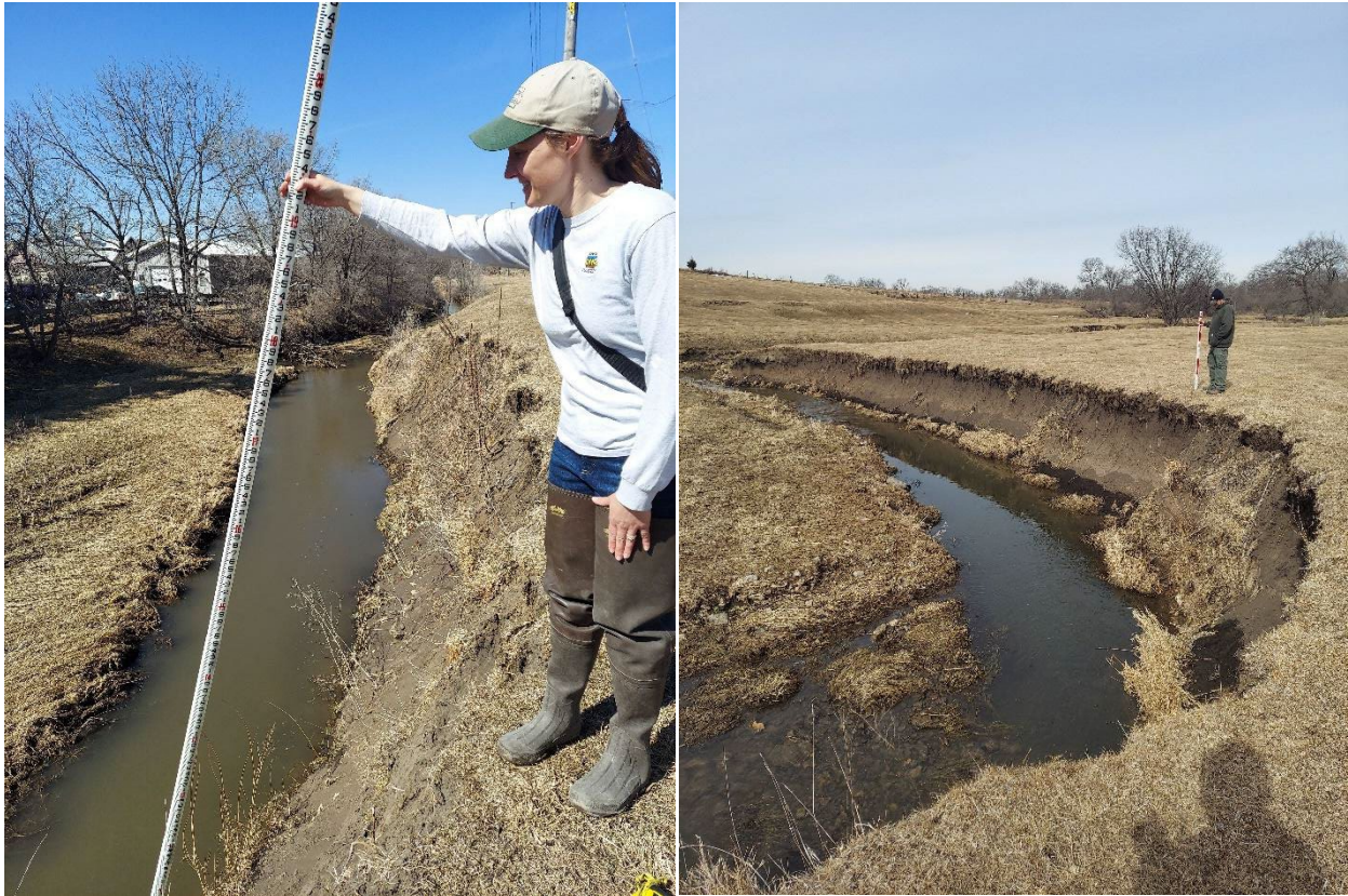
Figure 31. Moderate to severely eroded stream banks observed and measured during a RASCAL stream survey in the Trout Run Watershed.
